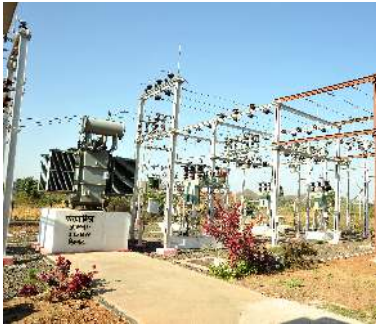
3.15 MVA, 33/11 KV Transformer
