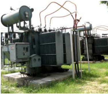
10 MVA, 33/11 KV Transformer
