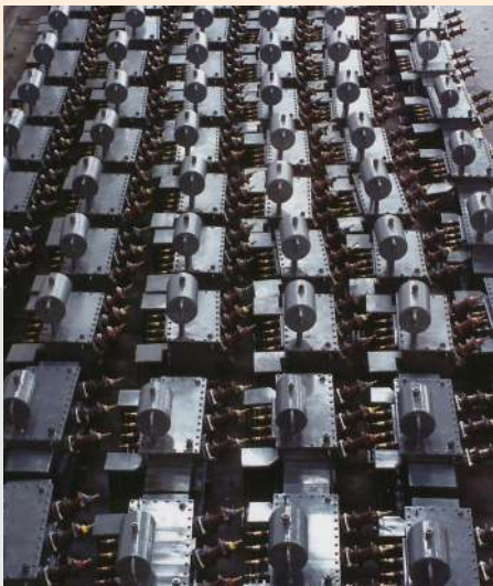
3 \phi Distribution Transformers (11 KV)
