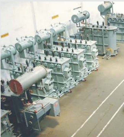
Power Transformer Bay
